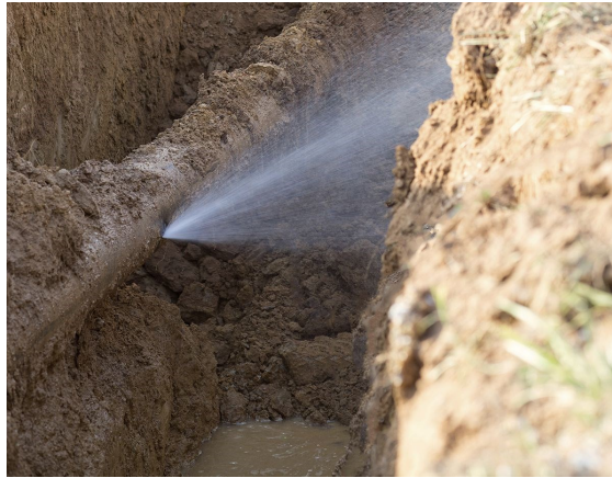
Buried distribution main leaks are a common contributor to lost and unaccounted for water.
